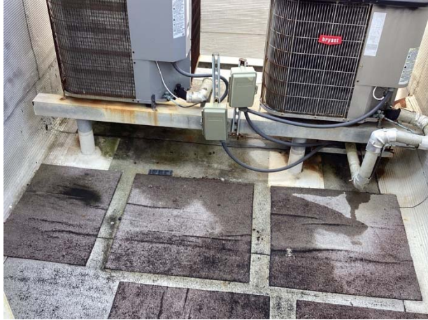
Standing water at lower roof
