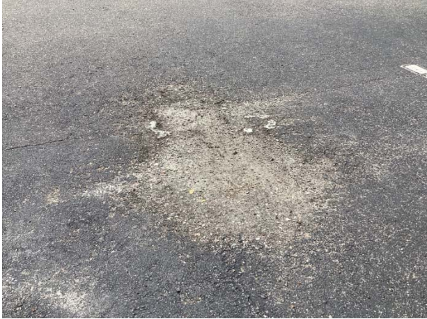
Area of significant raveling
