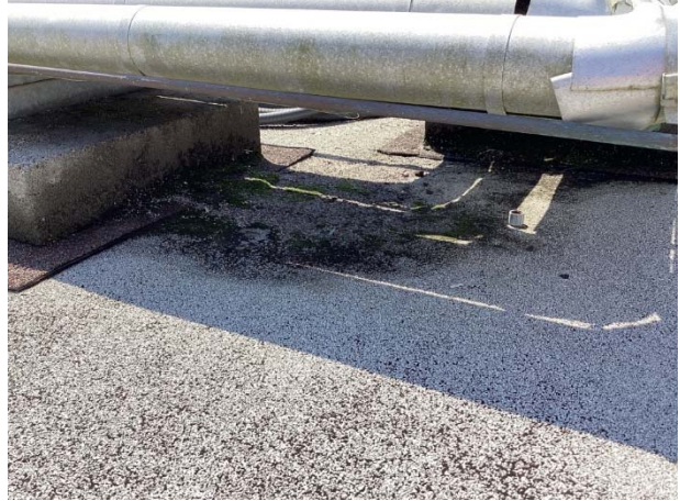
Stains beneath HVAC equipment
