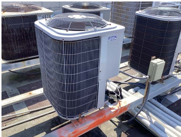
Split system condensing unit to club room
