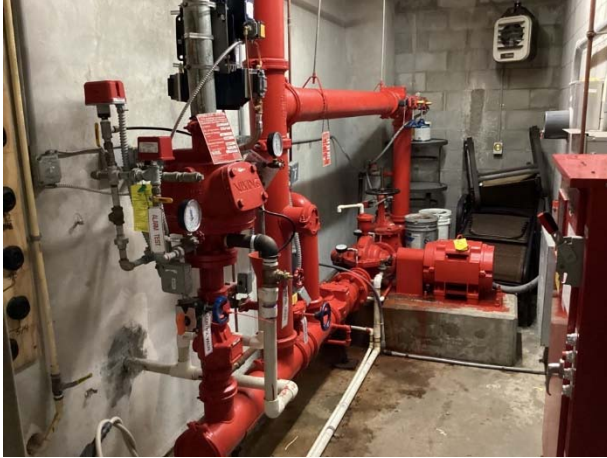
Fire suppression pump
