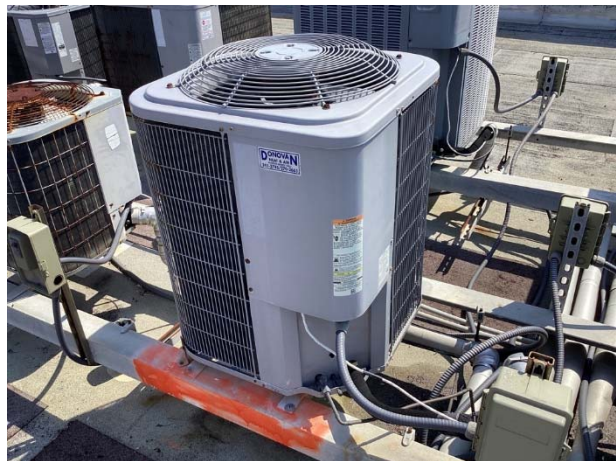
Fitness room condensing unit
