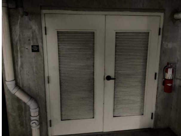
Pool mechanical equipment doors
