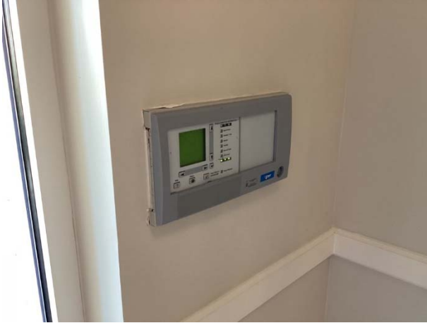
Lobby secondary panel
