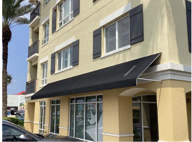
Awning with patch repair
