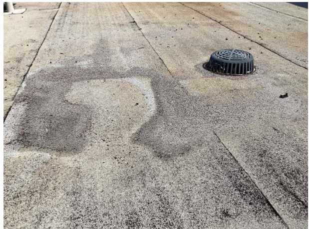
Granule accumulation at low spots
