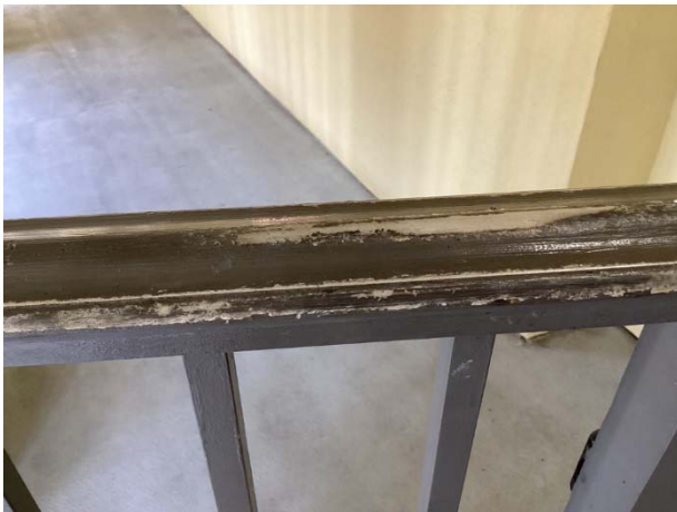
Finish deterioration at pool railing gate
