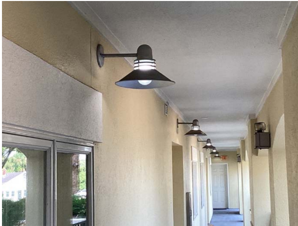
Exterior light fixtures
