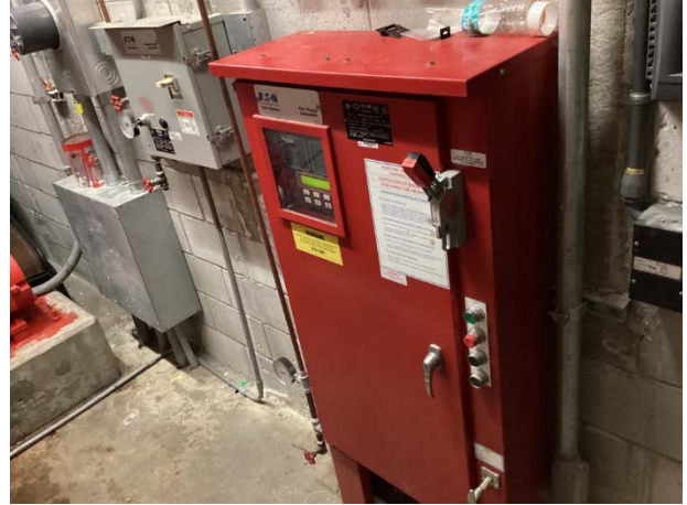
Fire suppression pump controls
