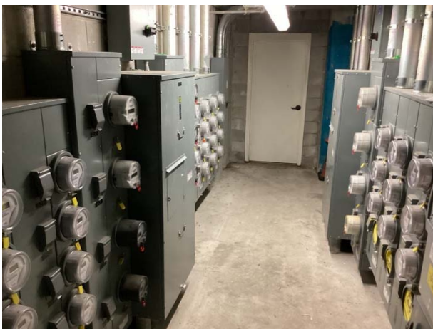
Electrical system components
