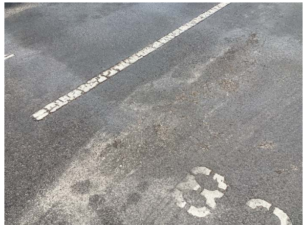
Area of significant raveling
