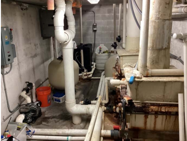
Pool mechanical equipment room
