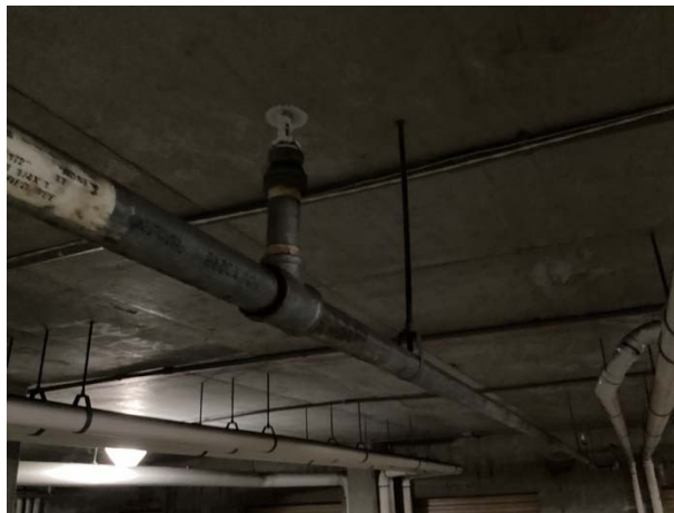
Fire suppression system
