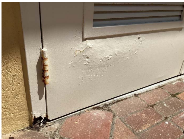
Corroded Doors at pool
