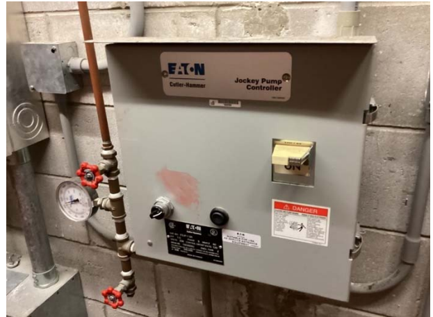
Jockey pump controls
