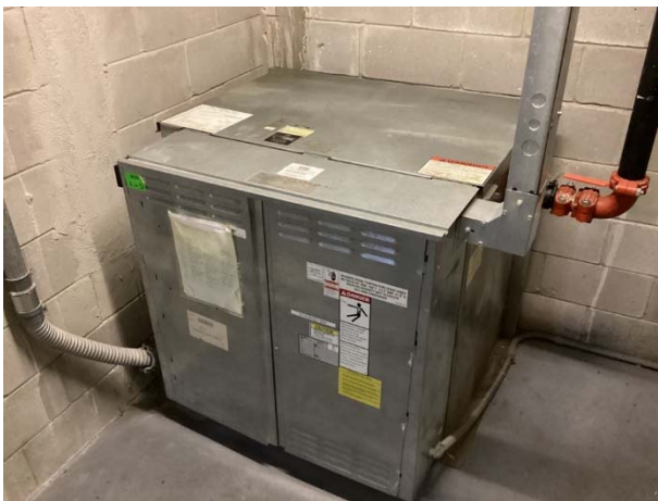
Hydraulic elevator equipment
