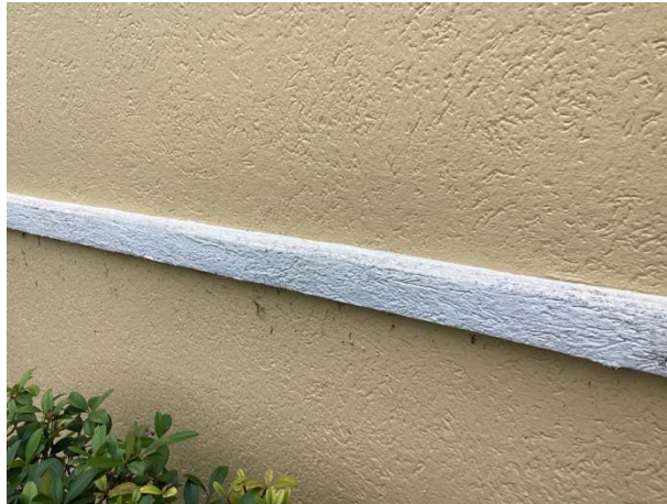
Isolated debris accumulation
