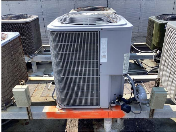
Lobby condensing unit
