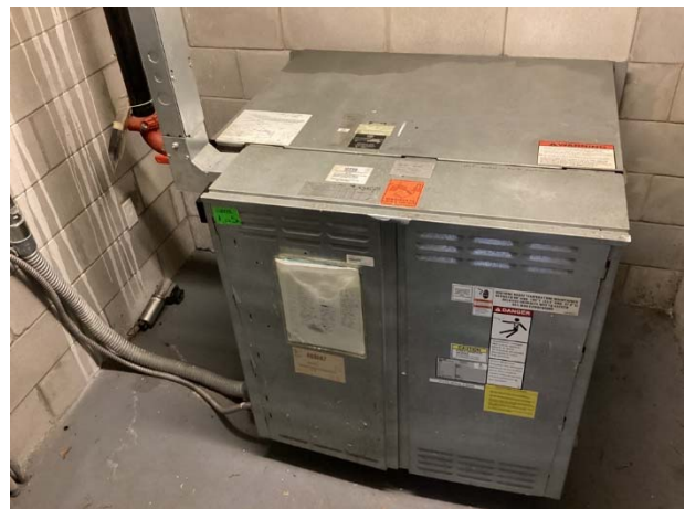
Hydraulic elevator equipment
