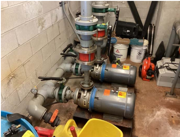
Domestic water pumps
