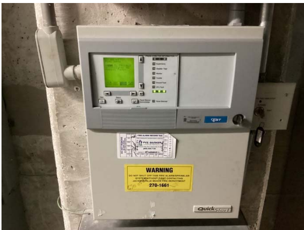
Control panel with trouble code
