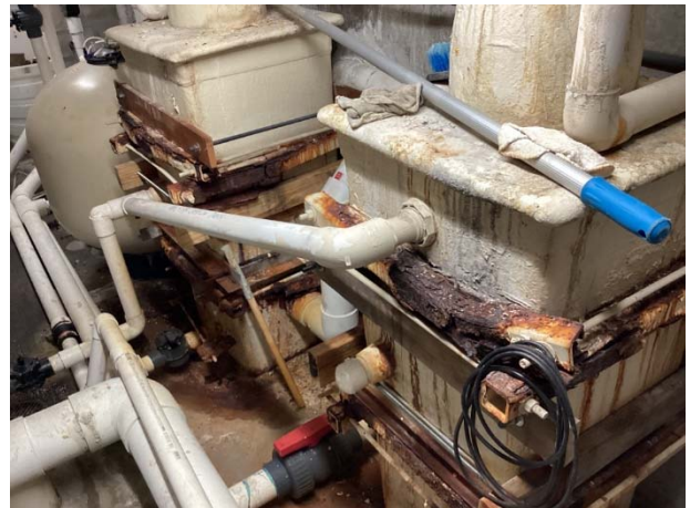
Significant corrosion at filtration equipment
