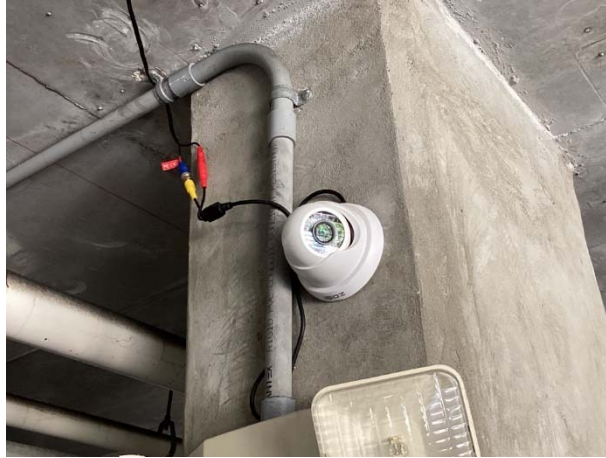
Security system camera
