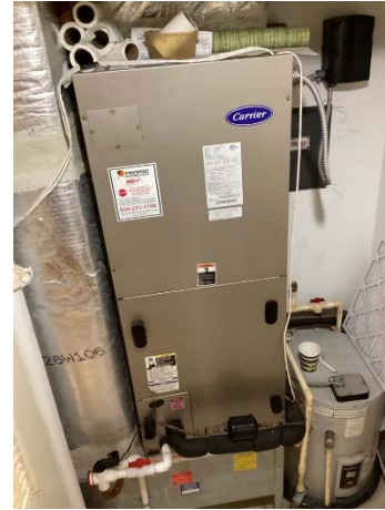
Split system air handling unit at pool rest room
